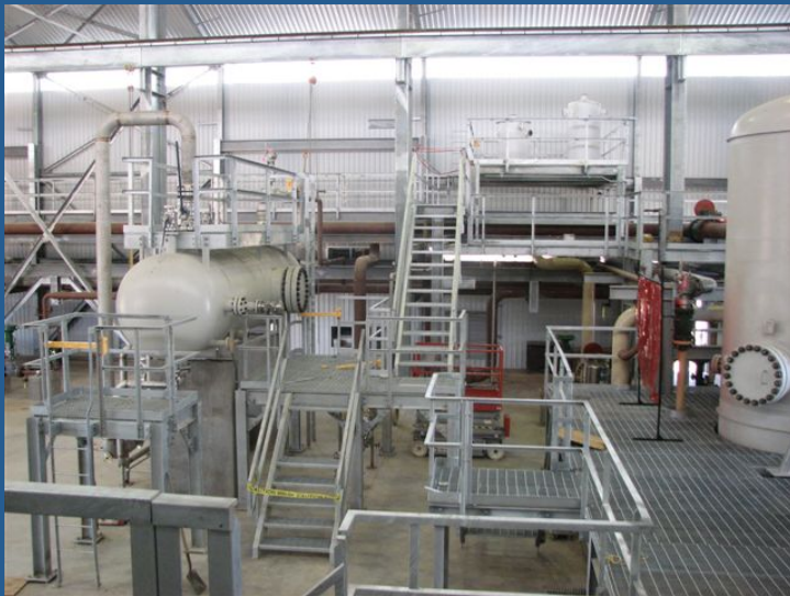
CO 2 Dehydration Equipment Colorado, U.S.A.
